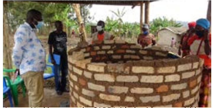
Aggrey Ntakimanya , the CARE Initiative Manager visiting Mandeleo Group in Kakoni at the site where they constructed a kiln for burning charcoal briquettes.
